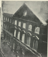
A PART OF THE HEAVILY DAMAGED BUILDING. THE BUILDING WAS HEAVILY DAMAGED BY THE GERMANS.
